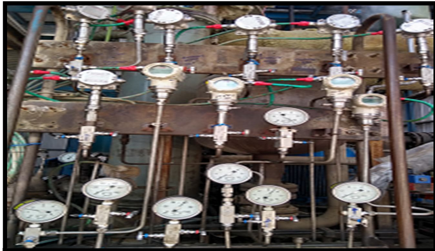
Main Air Blower Turbine Gauge Board Inst.
