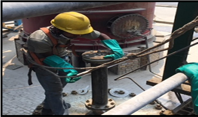
U-seal LT Removal for Cleaning & maintenance.
