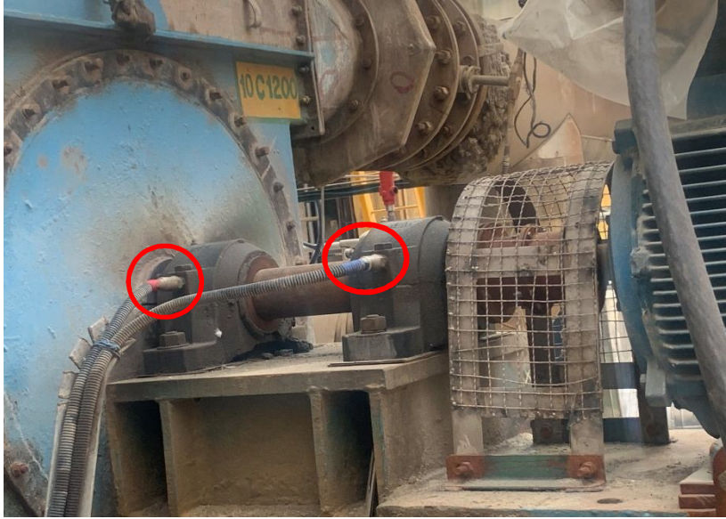
Fig 1.2(d) Vibration sensor arrangement in plumber block of PA fan
