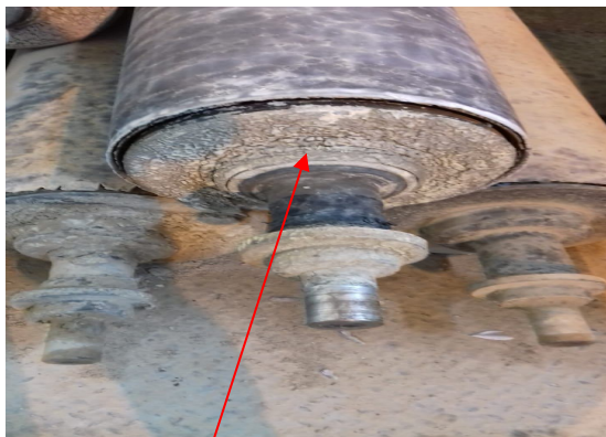
Damaged taken out Rollers
