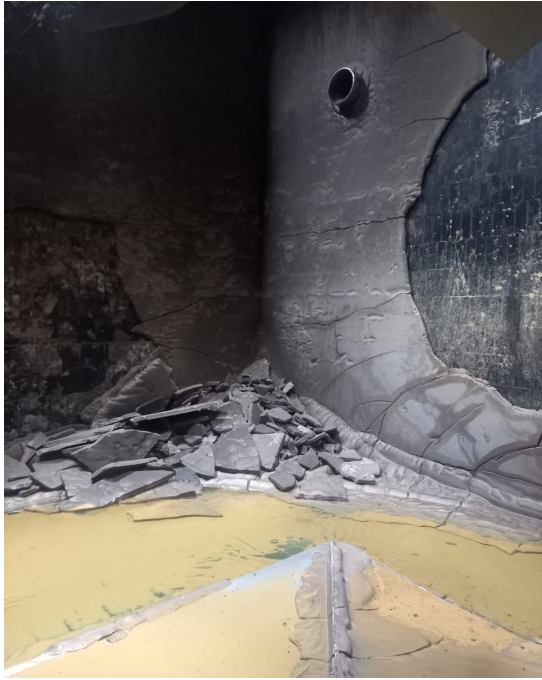
FFT wall before cleaning
