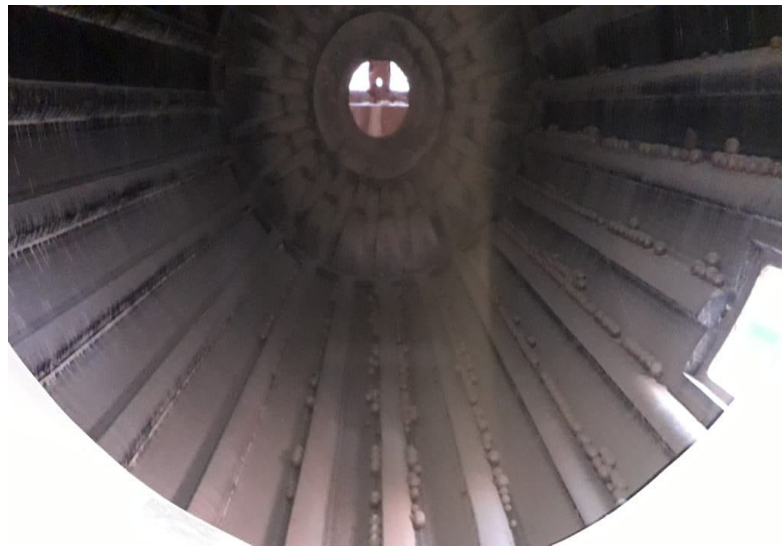
Ball mills water washed
