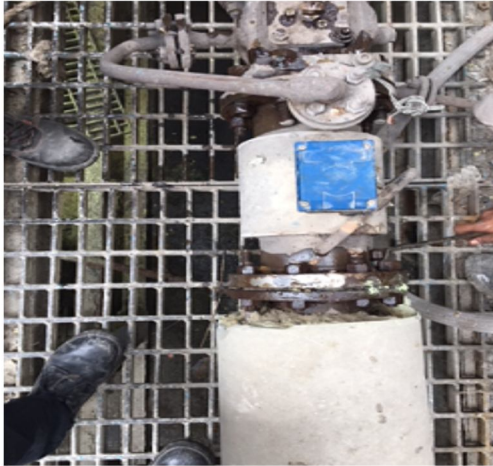
OLD Sulphur Flow meter
