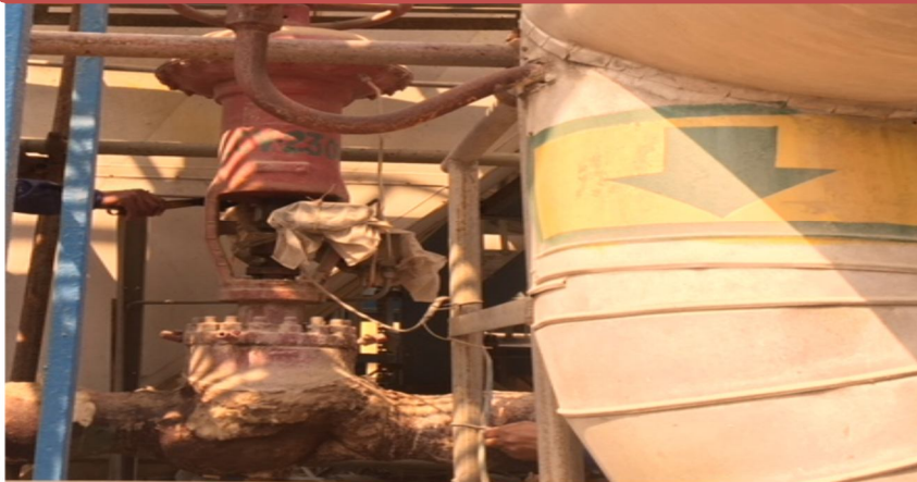
Old 10LCV1301 before Replacement
