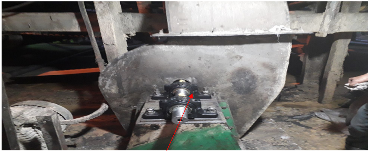
Air Suspension Blower after overhauling
