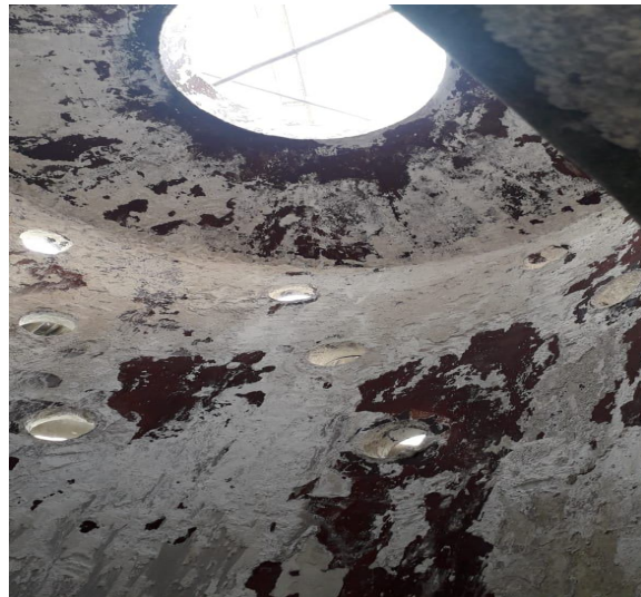
Pre scrubber inner shell after cleaning
