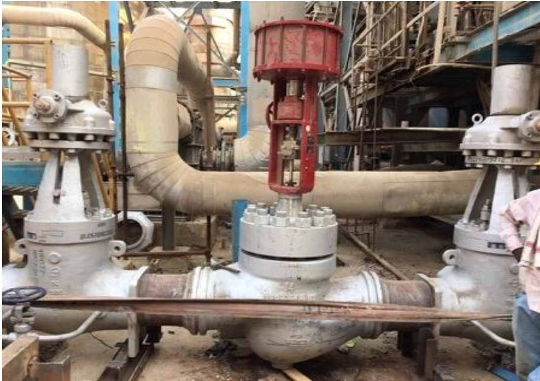
INSTALLATION OF CONTROL VALVE WITH ISOLATION VALVES
