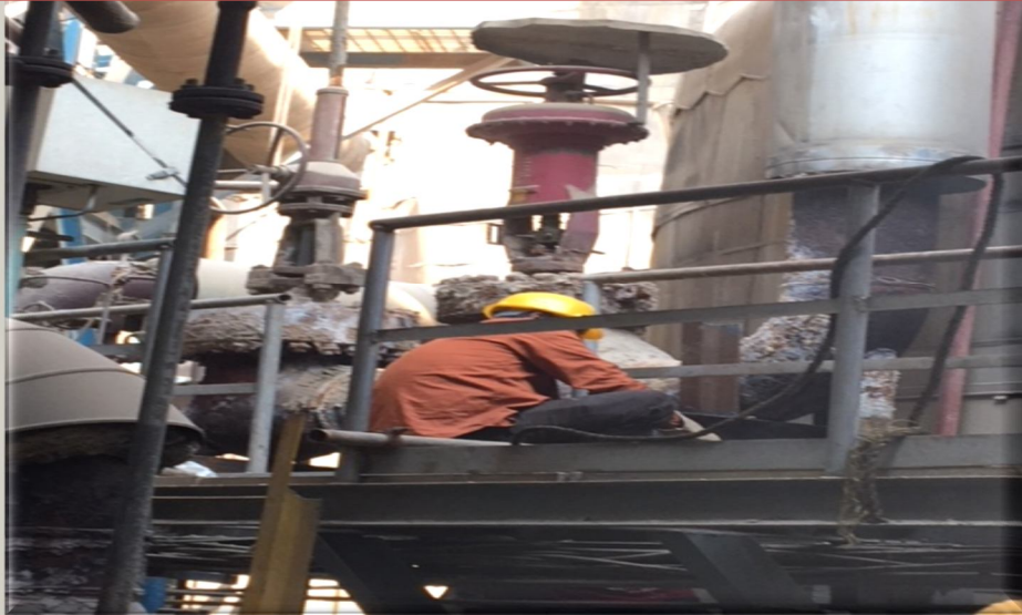
Old 3-Way 10TCV1506 before Replacement
