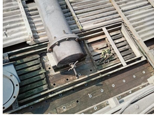
New FCV after installation
