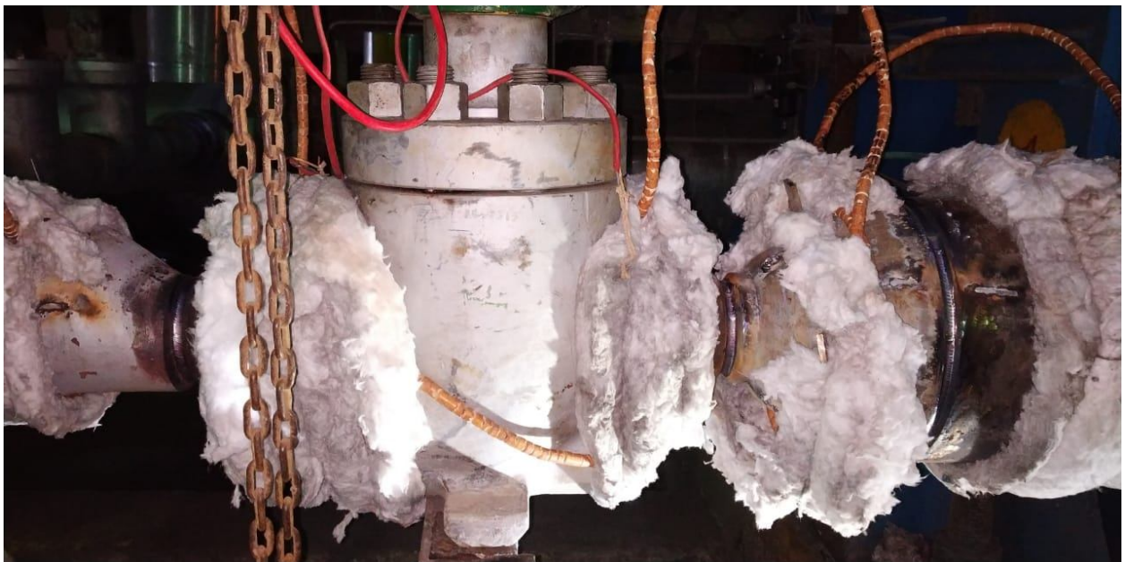
Figure 14: Root welding & hot passes completed and preheating for fill up & final welding
