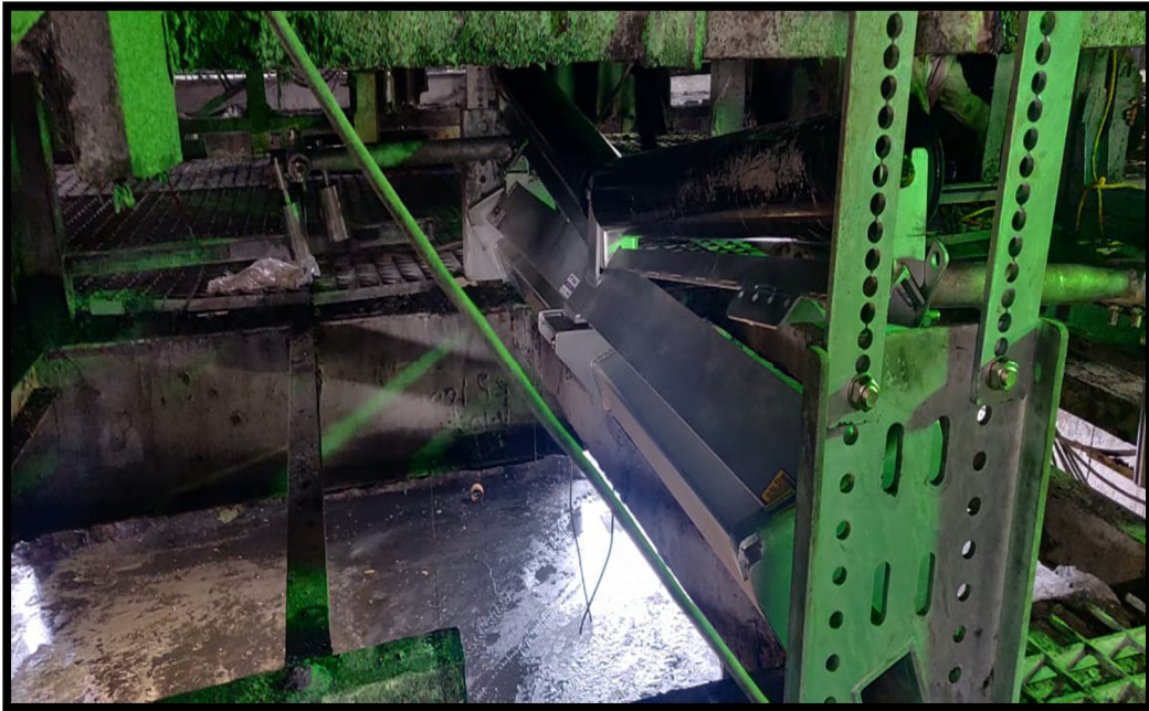
Fines Conveyor return belt tracker
