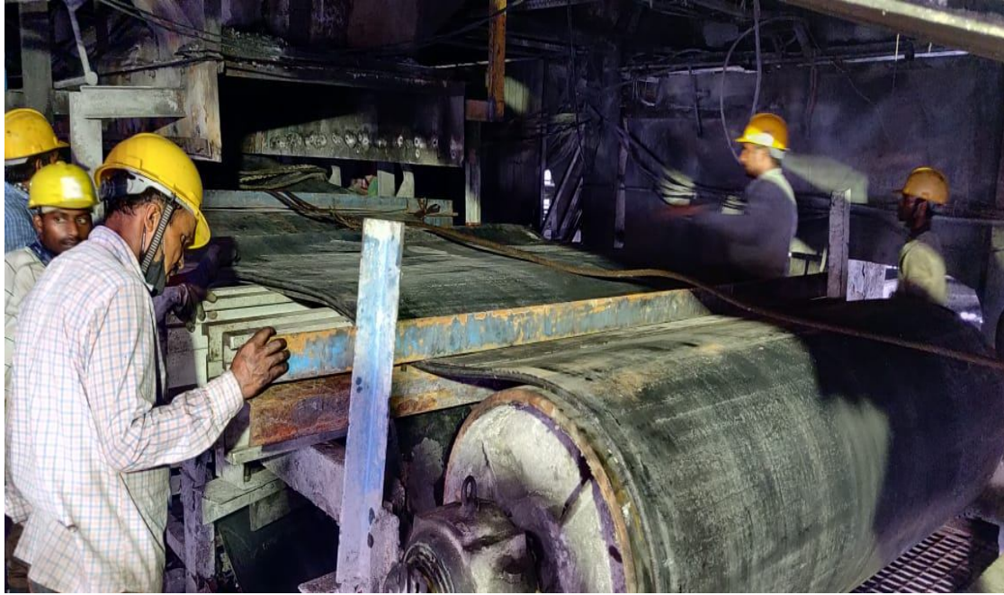
Fines conveyor splicing arrangement
