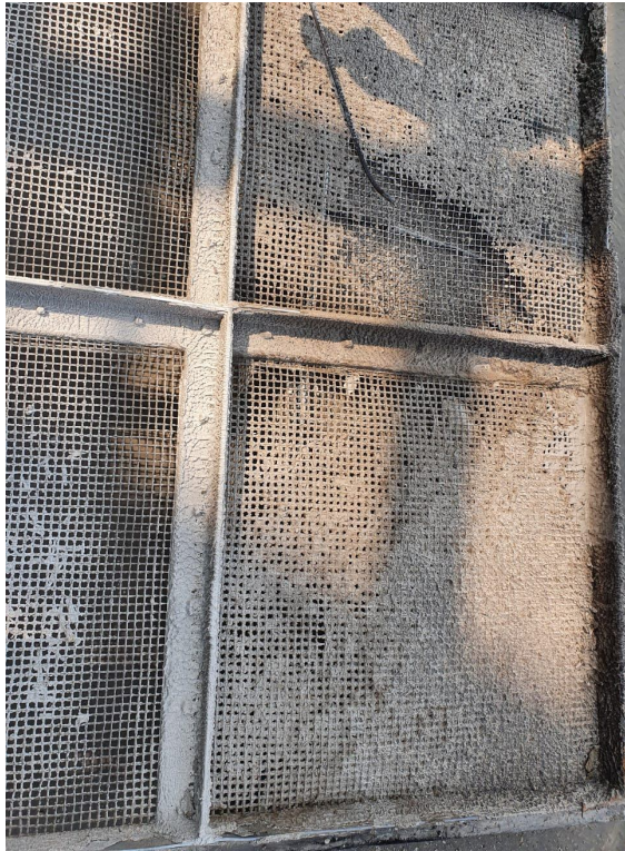
Cooling Tower Strainer before cleaning
