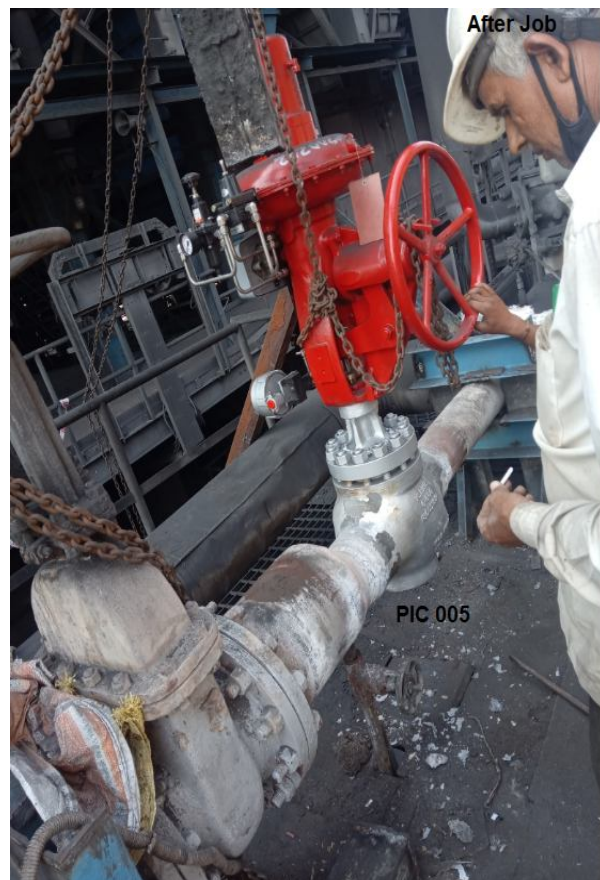
New Control Valve
