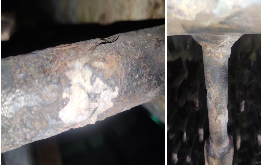
Header drain line was found corroded and was replaced
