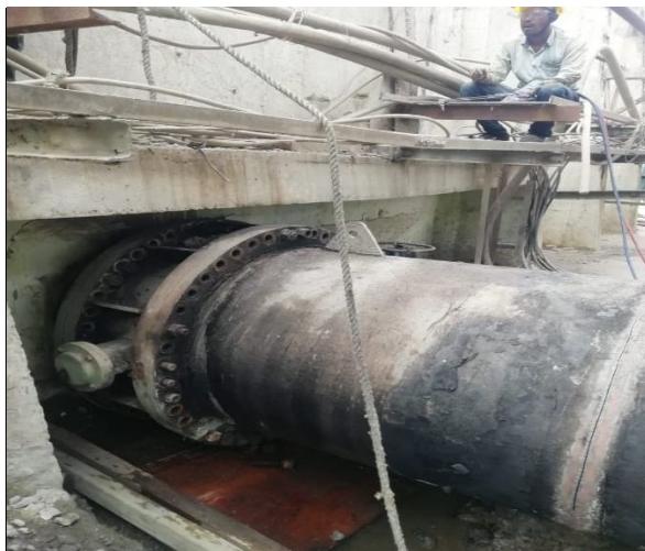
Suction Valve before Replacement
