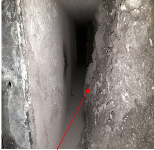
Chocked Air Duct
