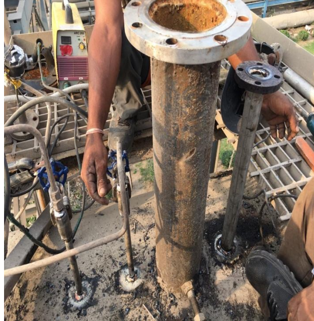
PH and Temperature nipple After Replacement
