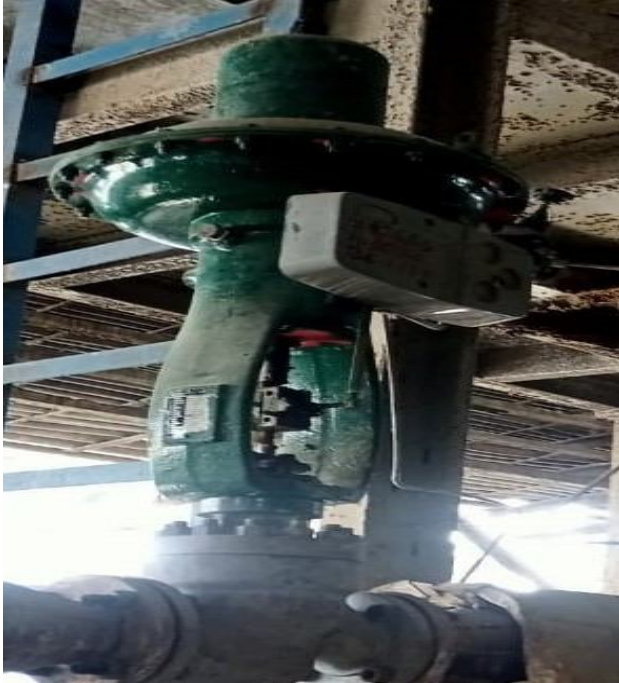
New M/s MIL make Control Valves in Filtration A & E.
