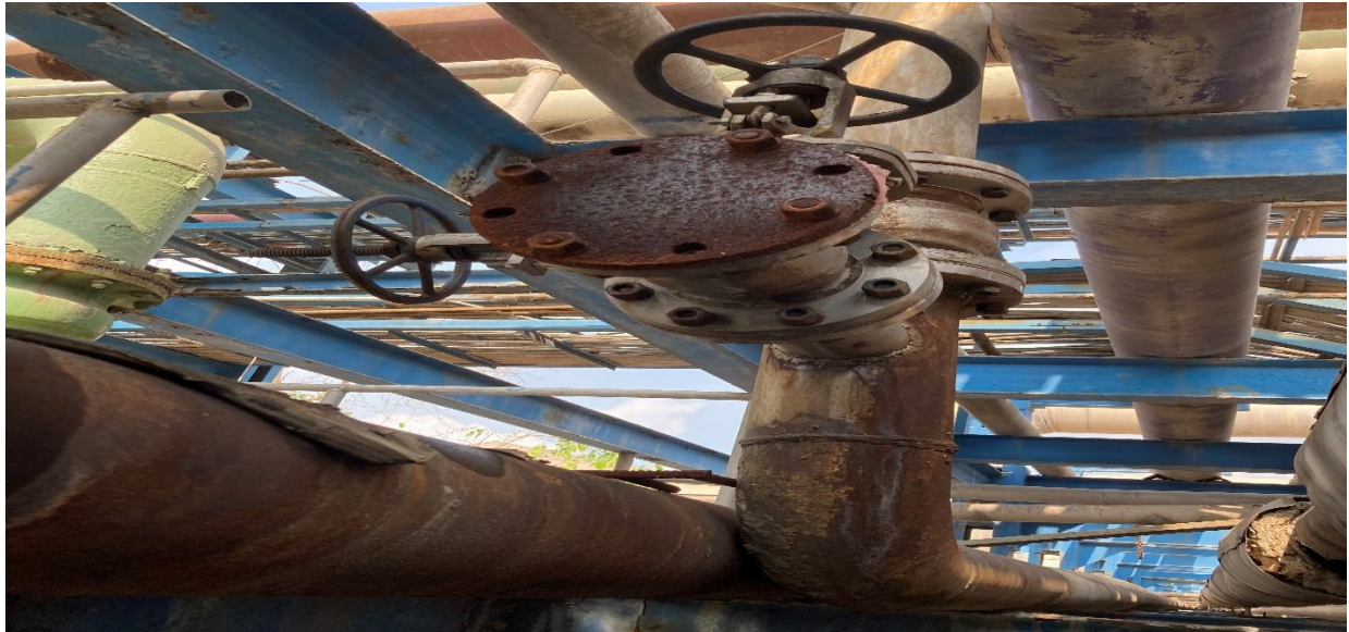
4" Tapping for Condensate Line
