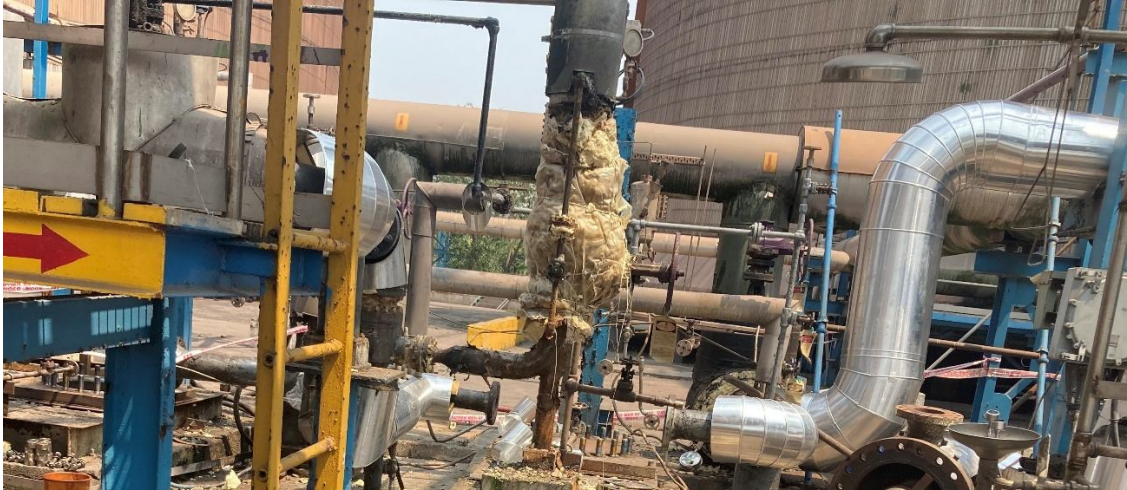
Insulation of 12" Ammonia suction and discharge line
