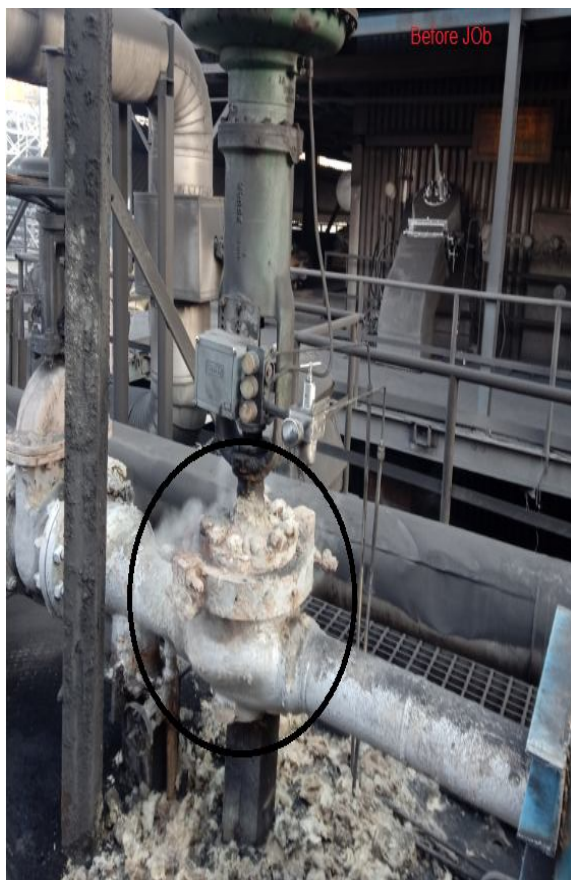
Old Control Valve
