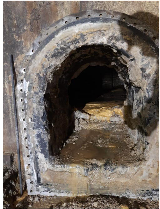
VCST manway after descaling
