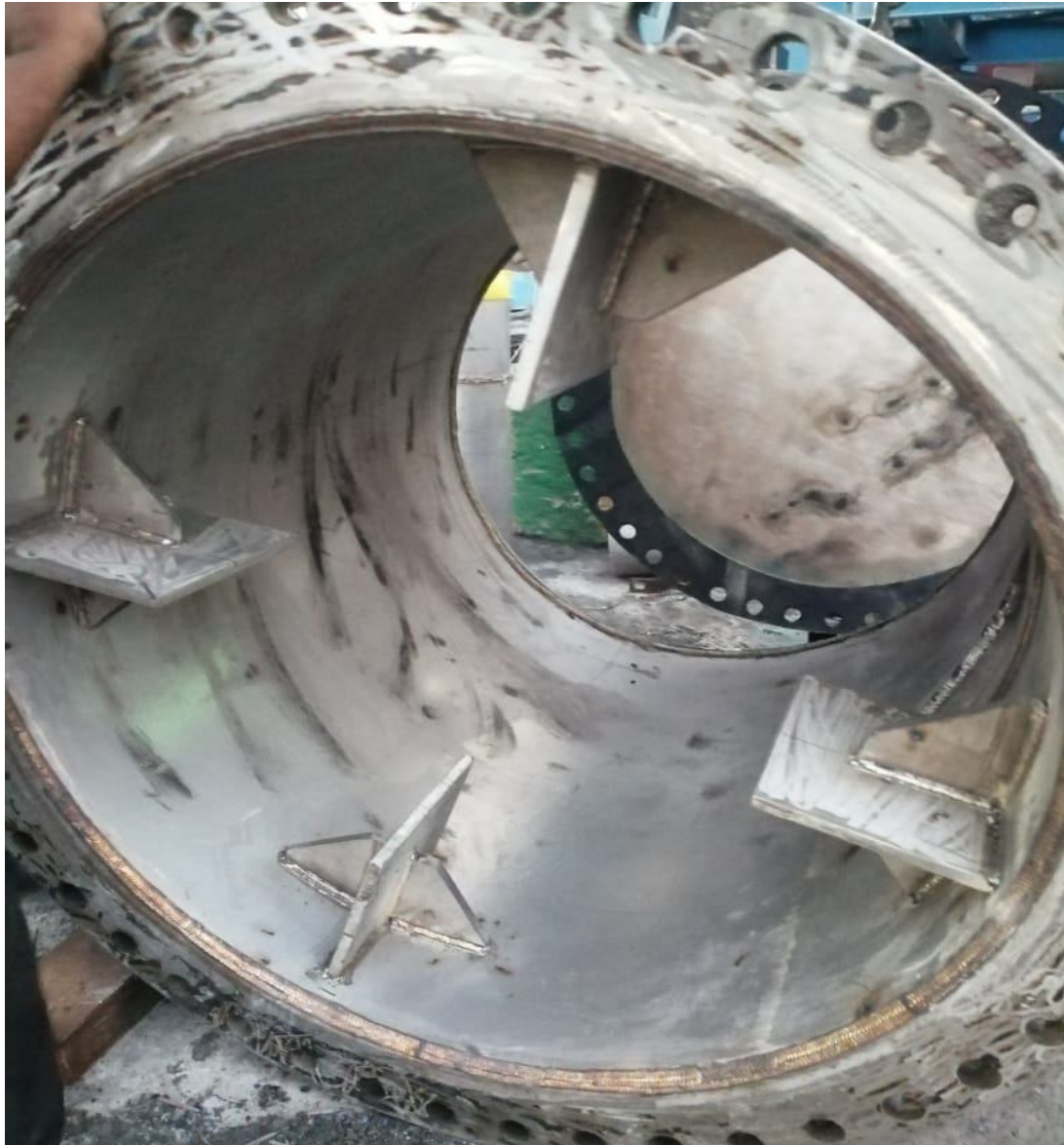
VORTEX BREAKER PROVIDED IN SUTION SPOOL PIECE IN (P-113) TO AVOID CHURNING IN THE PUMP
