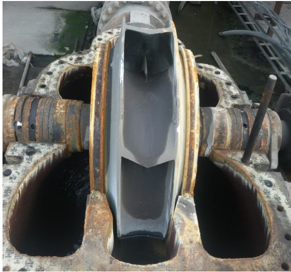
Fig: SAP cooling tower Pump B casing rotor condition.
