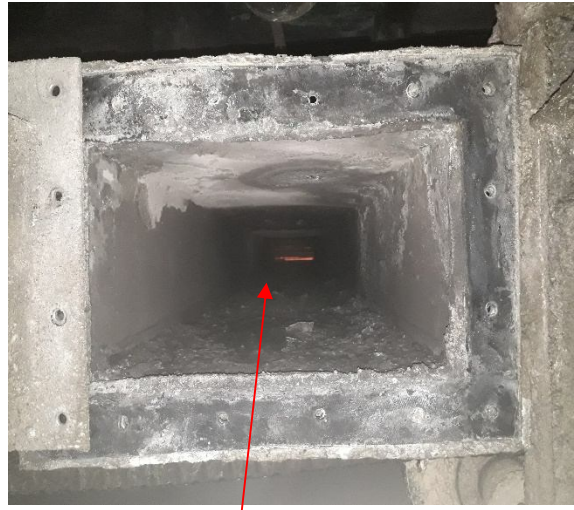
Air Duct after cleaning.
