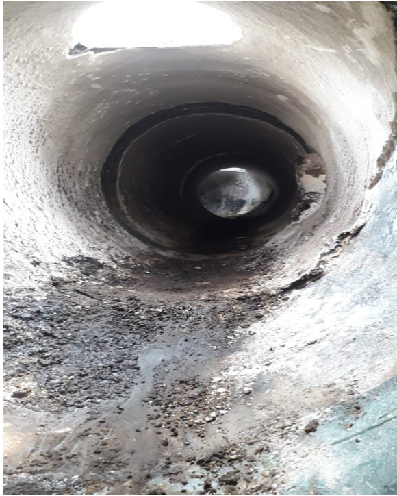
Fumes duct before cleaning
