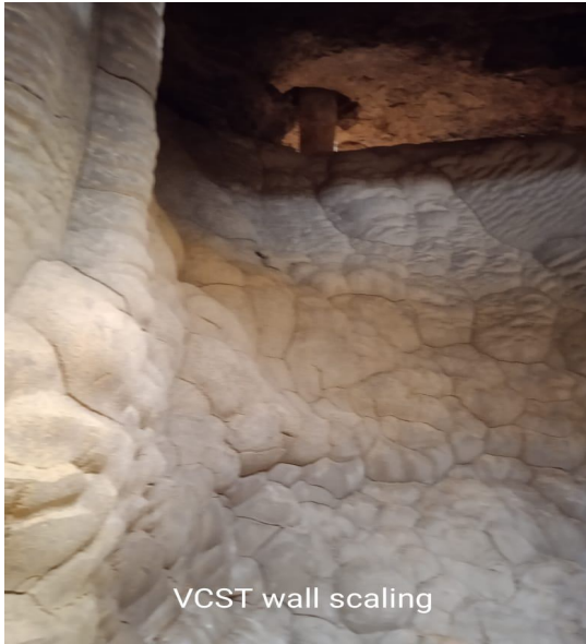
VCST wall before cleaning
