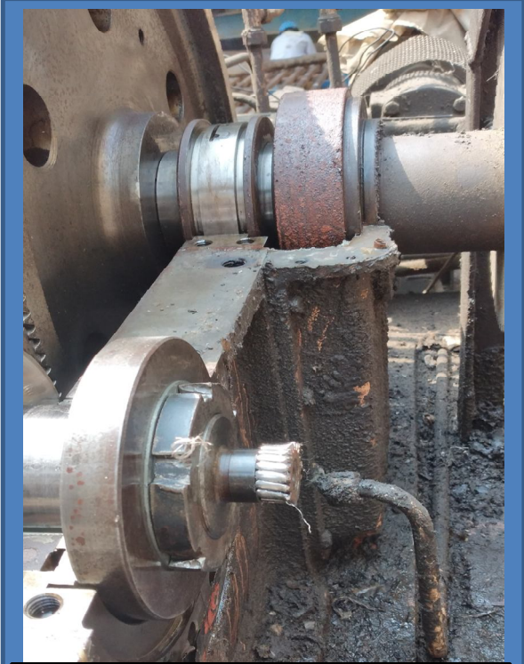
BFW 101C GOVERNOR PINION FOUND DAMAGE
