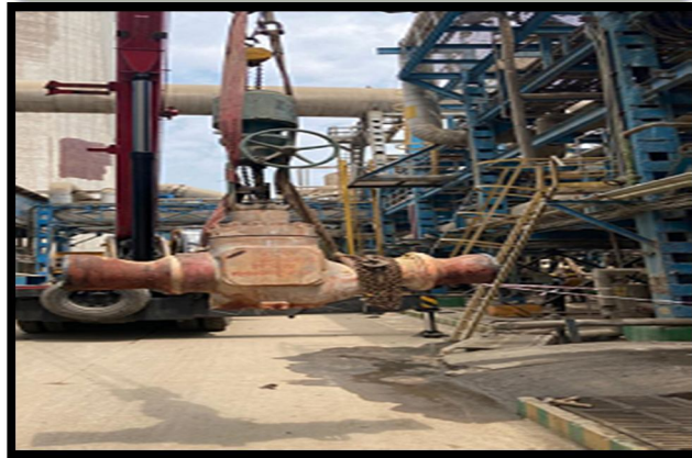
Old PCV-1555 Control Valve
