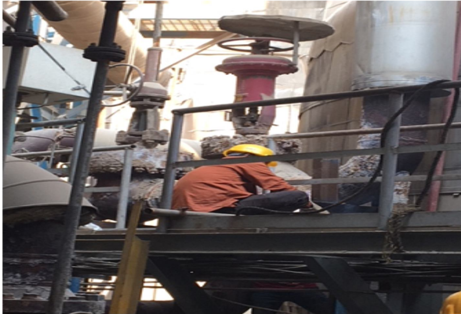
OLD 3-Way Control Valve 10TCV2506
