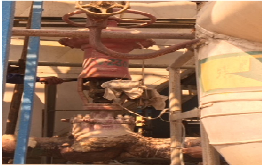
OLD Drum level Control Valve Tag 10LCV2301
