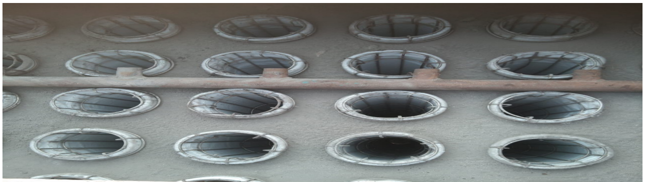
NEW BAGS WITH SS CAGE FITED INSIDE THE VENT FILTER BOX
