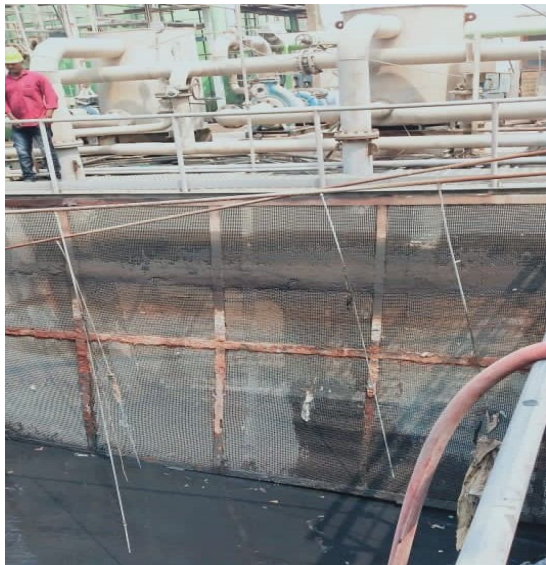
Neutralization Pit Pump Suction strainer before.
