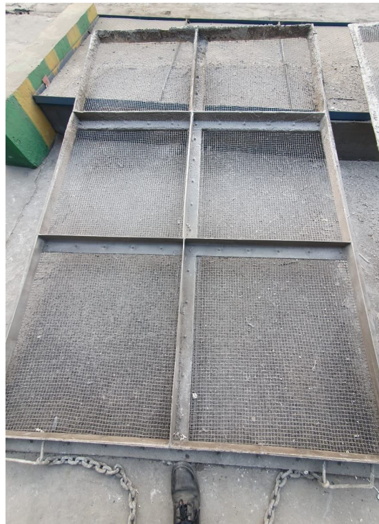
Cooling Tower straner after cleaning
