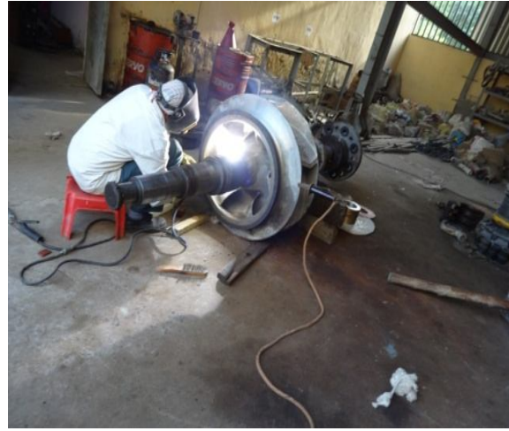
Rotor Assembly Condition after cleaning
