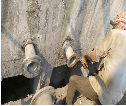
S.S. pipe and flange fitting
