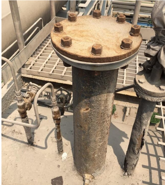
PH and Temperature Nipple before Replacement
