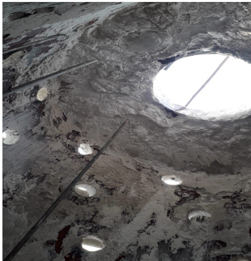
Pre scrubber inner shell before cleaning
