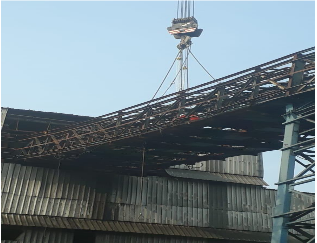
SAGGED PORTION OF GALLERY- BC- 130 /132 – BAGGING PLANT
