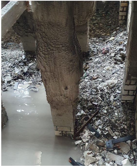
Old Cooling Tower Cell before cleaning
