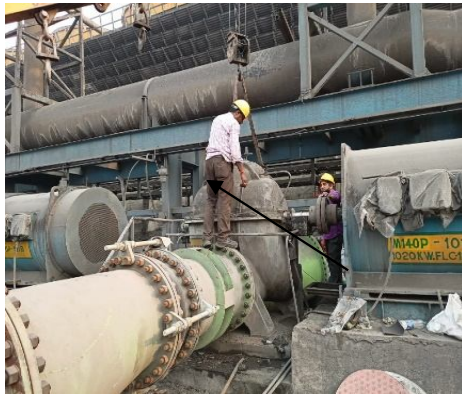
CASING BOX UP OF TG CT PUMP 'C'
