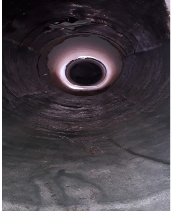
Fumes duct after cleaning
