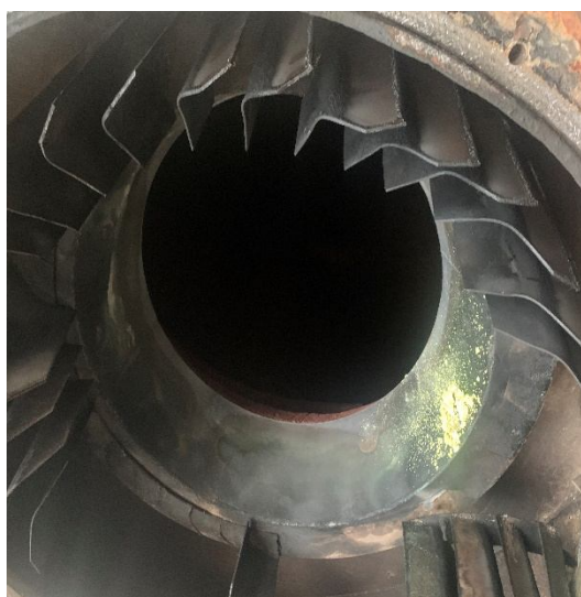
Fig 1.1(a) damaged vane of air resister
