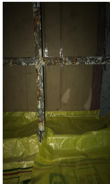
Covering of tubes & header
